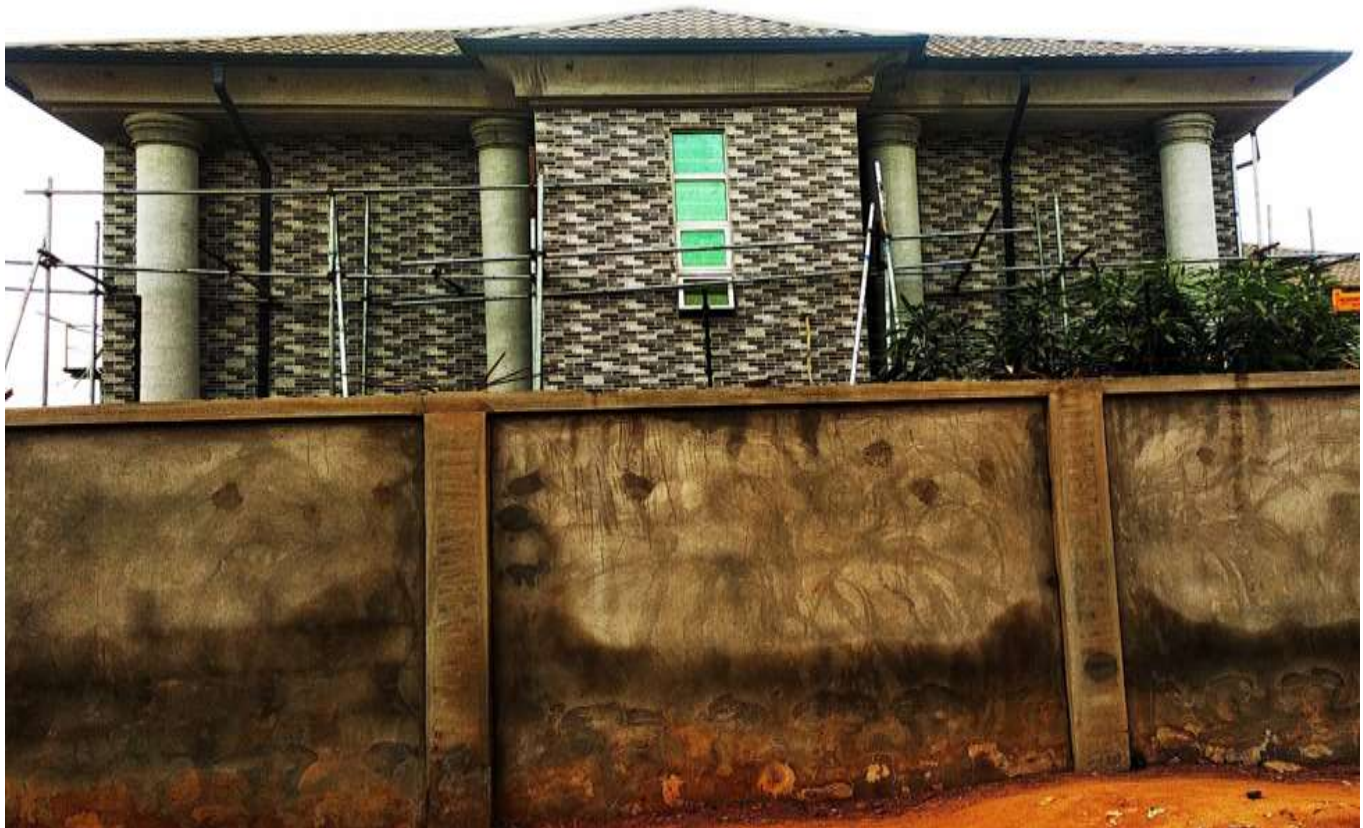
Figure 3: A Building and its Perimeter-fence constructed with Sandcrete masonry blocks as the major walling-material. However, while the Perimeter-fence is only plastered with mortar, Ceramic tile is used for the exterior finishing of the Building
