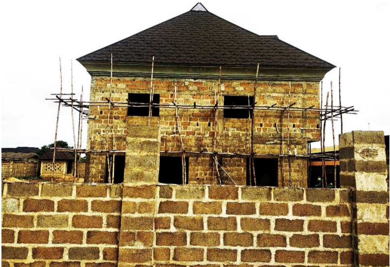
Figure 1: A Building and its Perimeter-fence under construction with the use of Sandcrete masonry blocks as the dominant walling-material
