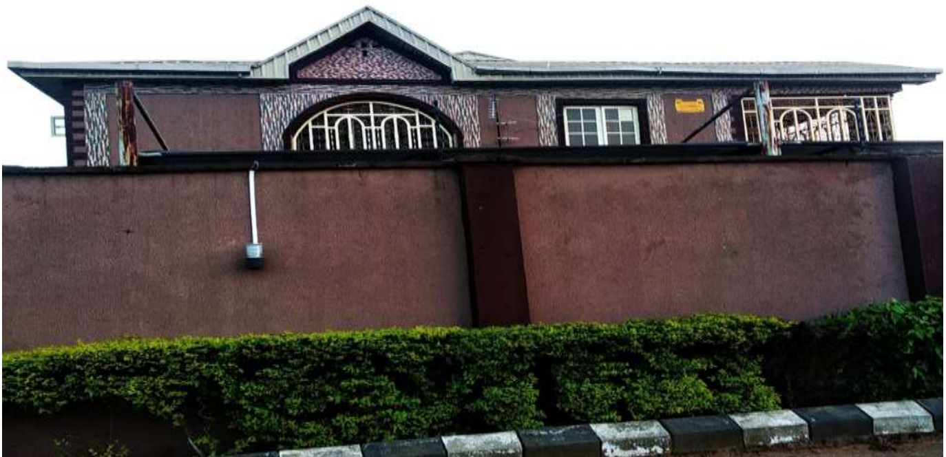
Figure 5: A Building and its Perimeter-fence constructed using Sandcrete masonry blocks and plastered with mortar; with landscaping (kerb stones and flowers etc.). Moreover, while the exterior finishing material of the Perimeter-fence is only paint; while the exterior finishing materials of the building are paint and ceramic-tiles
