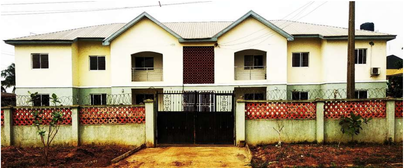
Figure 4: A Building and its Perimeter-fence constructed with Sandcrete masonry blocks and plastered with mortar. In addition, the exterior finishing material of both the building and Perimeter-fence is paint; and the top courses of the Perimeter-fence are constructed with fired-bricks hollow fancy-blocks
