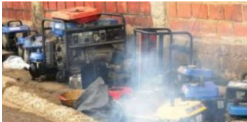
Figure 3- 1 Exhaust emissions from industrial generators [14]
