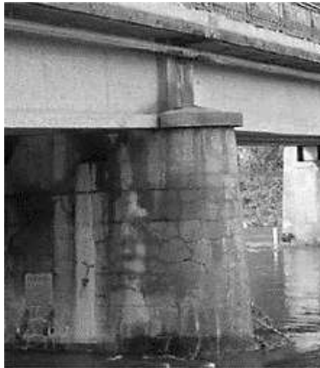
Fig.1 Cracking pattern in a bridge suffering from endogenous sulphate attack [9].
