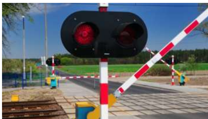
Figure 4: Red and white stripped boom gate with traffic lights
