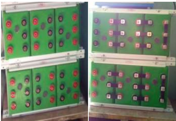
Fig 5: Sets of three (3) Batteries racked.
