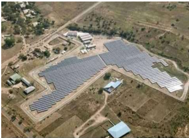
Figure 2: Project site showing PV installation on the MMS
