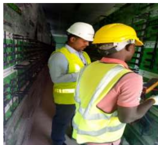
Fig 6: batteries connected in strings
