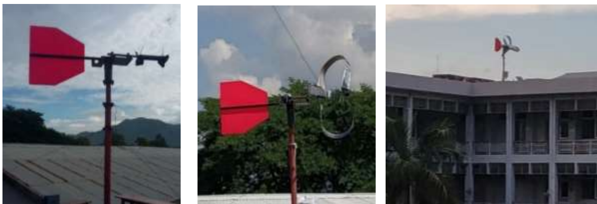
(a) Assembly of Hub, Shaft, Tail Vane (b) Assembly of LWHAWT (c) Assembly of LWHAWT at MTU
