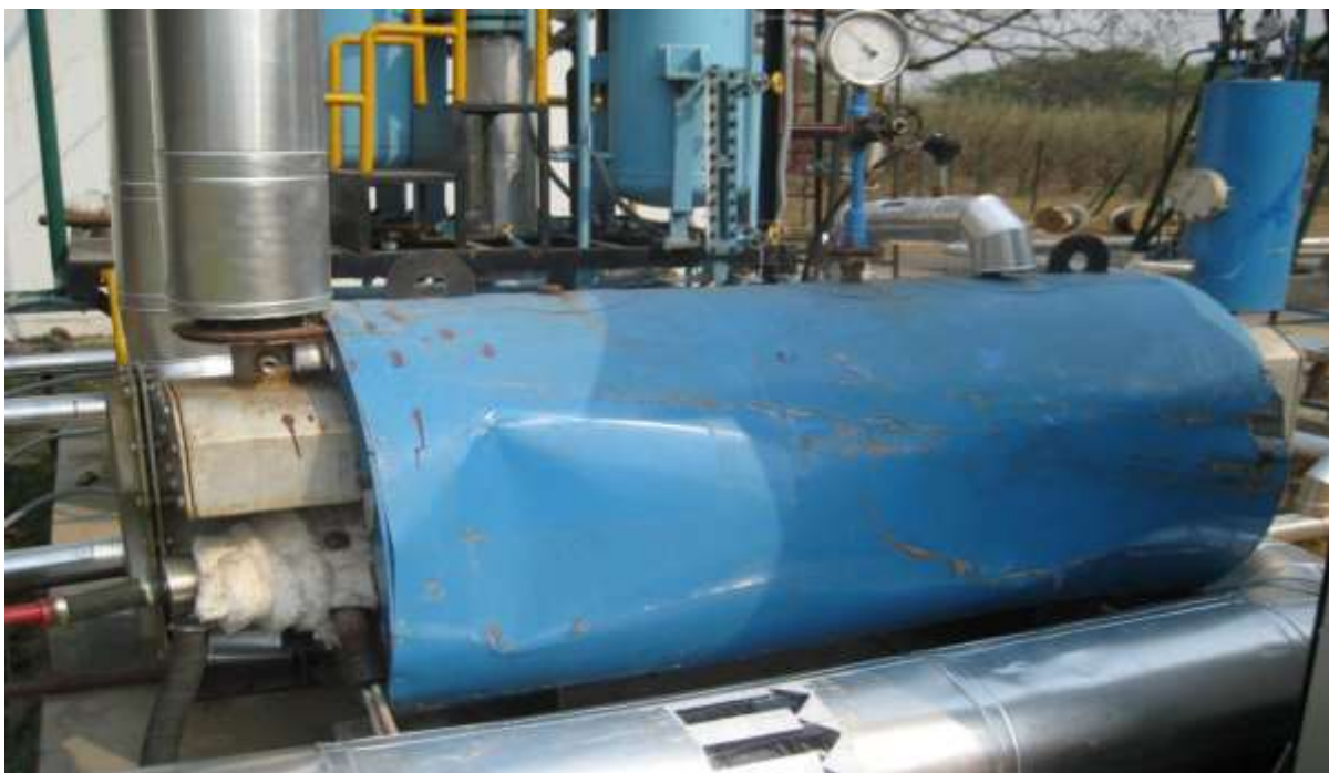
Figure 2. Plate No. 2 Waste Heat Recovery Unit
