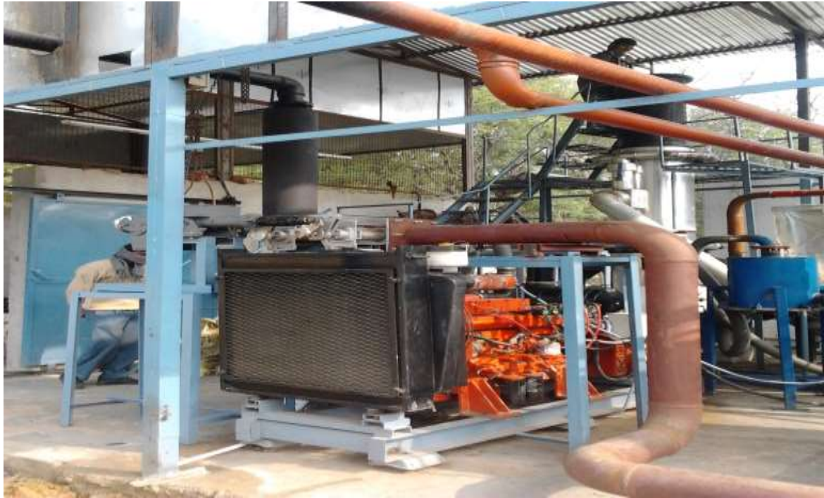
Figure1. Plate No. 1 Gas-Engine Generator
